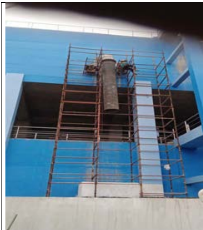
Figure 11: Safe Inlate pipe laying above 3rd floor slab of admin building in SD30R
