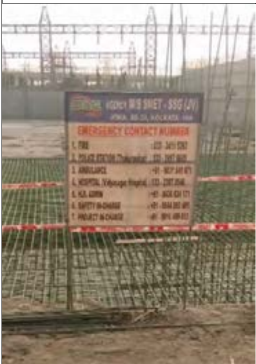
Emergency contact number display at site
