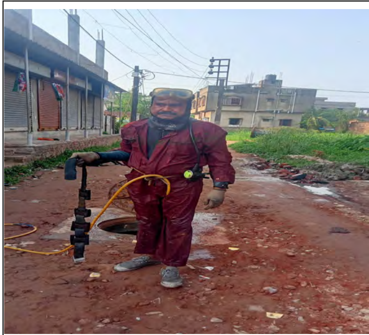
Seal Breaking work (Maintaining proper PPEs and safety measure) in progress at Rania (SD-10T)
