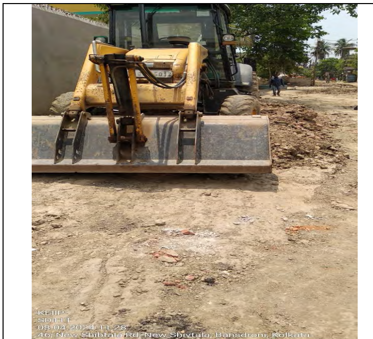
After pipe laying back filling and Rolling work in progress at Bramhapur (SD-11T)
