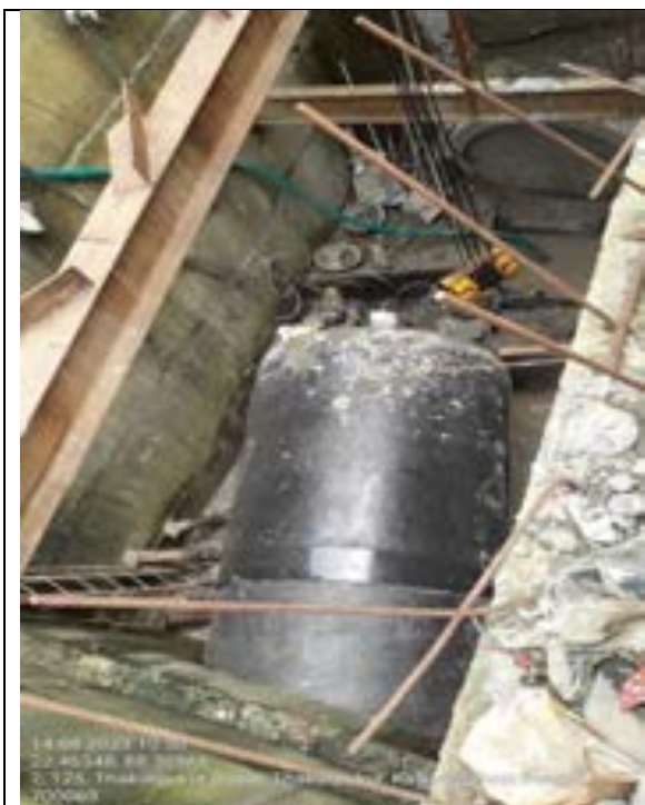
Figure 13: RCC pipe is being laid by microtunneling method at Thakurpukur Bazar in SD 31R2
