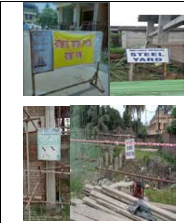
Safety caution board at project site
