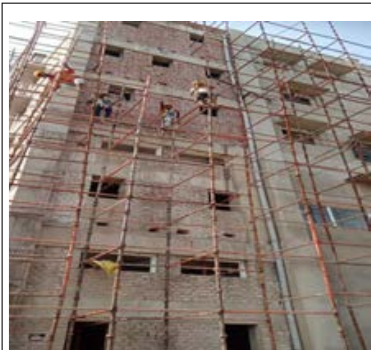
Figure 11: Casting of columns above 3rd floor slab of admin building in SD30R
