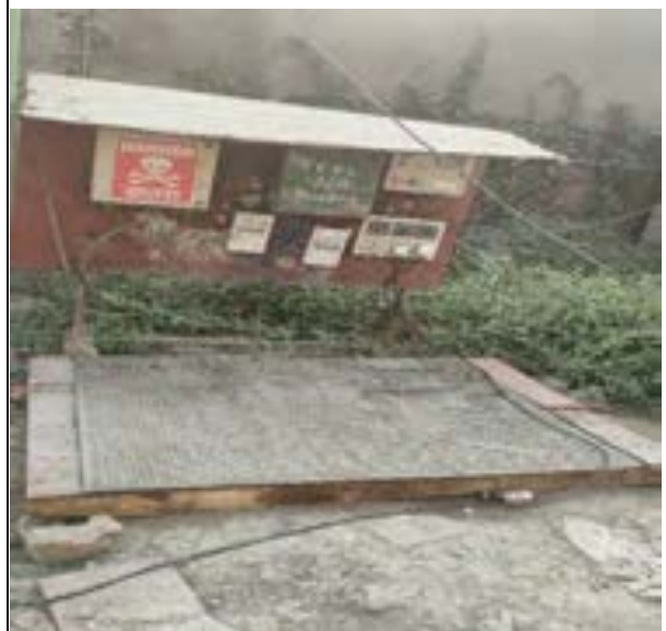
Rubber mat used in front of main panel board
