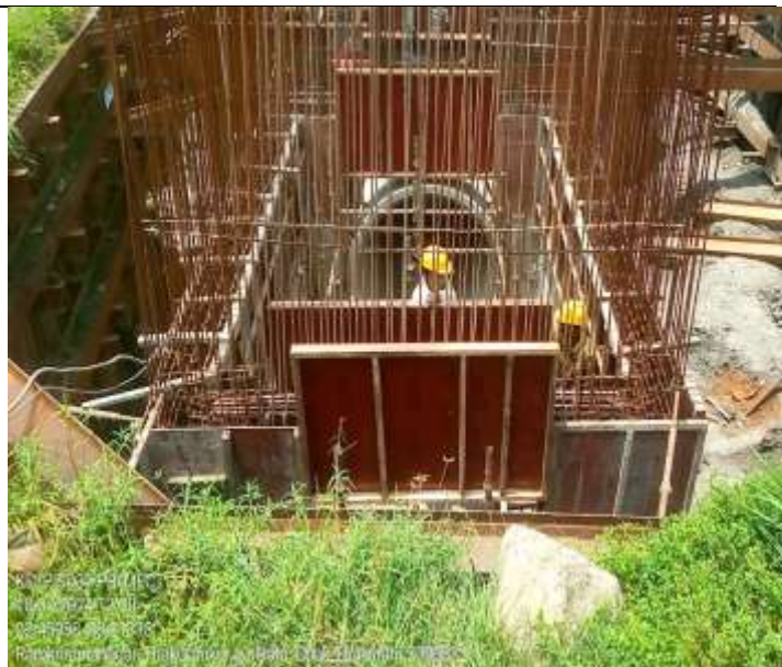
Figure 12: Launder base slab shuttering & reinforcement work are under progress in SD 31LOT1
