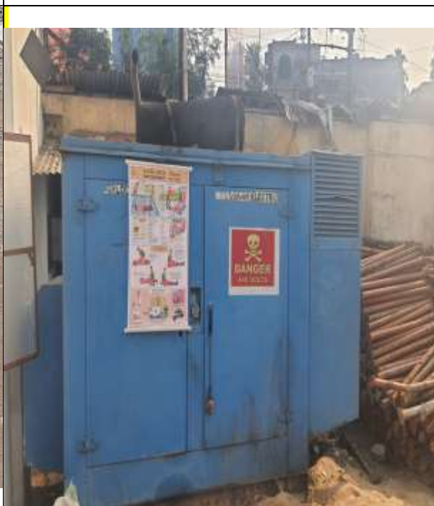
Alert Posters on Electrical Equipment
