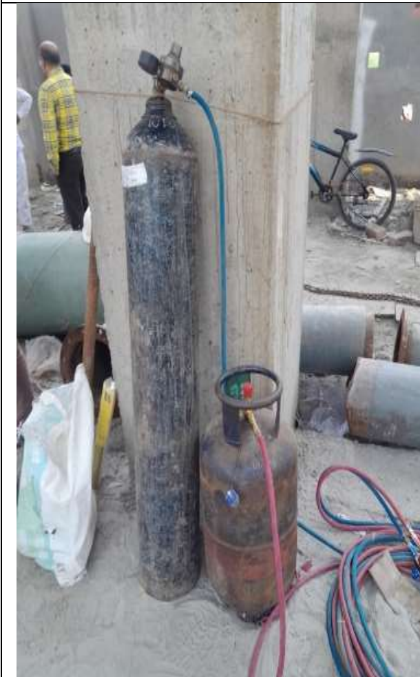
Secure cylinders in an upright position
