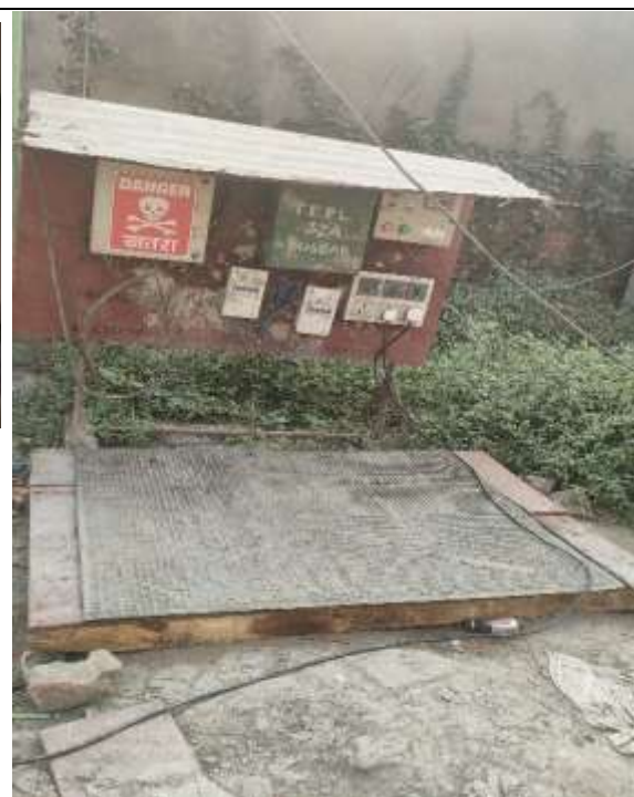
Rubber mat used in front of main panel board
